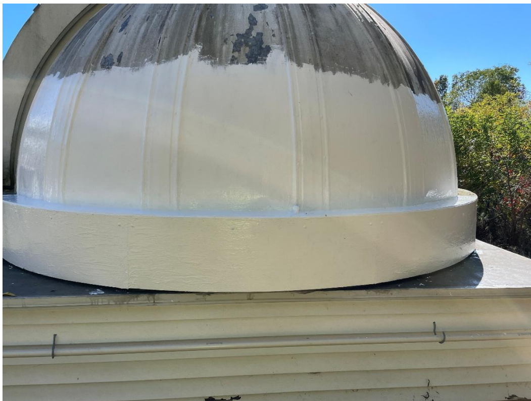
(above) Adding Flexseal to protect the Tinsley dome from weathering (in process). Credit: Roger McDonough
